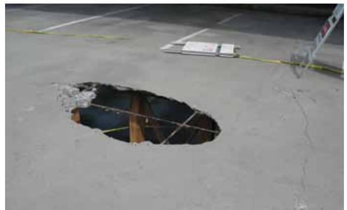
Fig. 2: Cracked and partially collapsed concrete slab showing exposed post-tensioning strands
