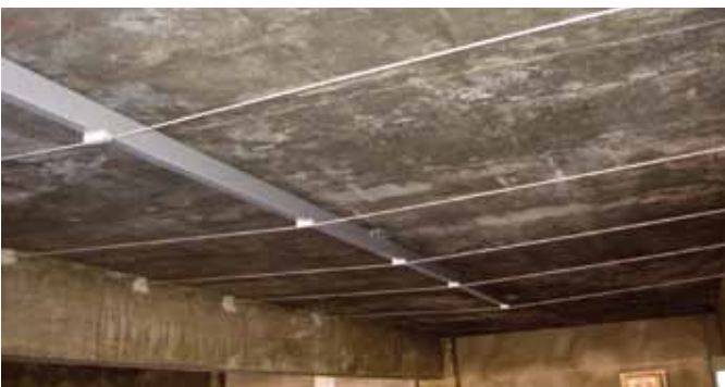
Fig. 7: HSS deviators were fastened to the slab soffit at the midspan of the slab. Post-tensioning strand traversed the beam webs near the slab soffit elevations and passed below high-density polyethylene saddles at the HSS
