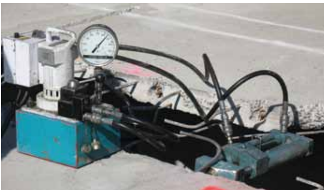
Fig. 10: Reseating an existing tendon anchorage. A slot for an external tendon is visible behind the pump
