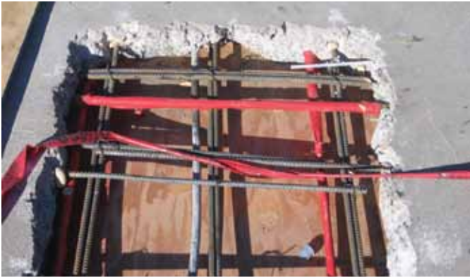
Fig. 9: In areas with severe damage, unsound slab concrete was removed and replaced. Here, reinforcing dowels have been anchored into the existing slab and exposed strands have been wrapped to prevent bonding with the new concrete
