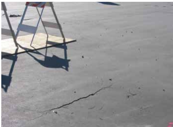
Fig. 3: Slab cracking at the edge of a supporting transverse beam below
