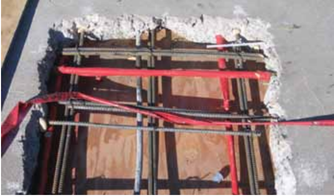
Fig. 9: In areas with severe damage, unsound slab concrete was removed and replaced. Here, reinforcing dowels have been anchored into the existing slab and exposed strands have been wrapped to prevent bonding with the new concrete
