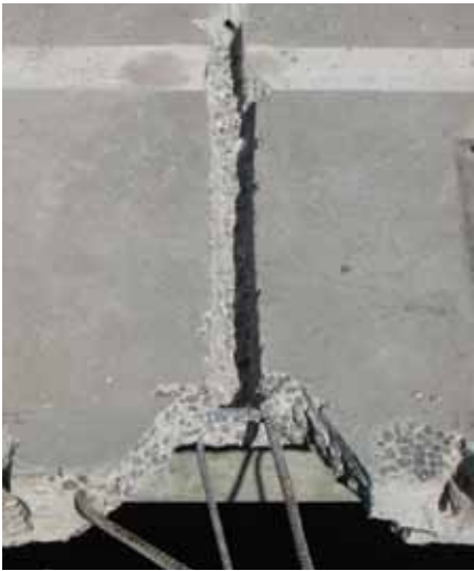
Fig. 5: Existing tendon anchors (lower right) were exposed to allow reseating. Here, a slot has also been provided to allow an external tendon to be anchored at middepth of the slab, near the existing tendon anchors
